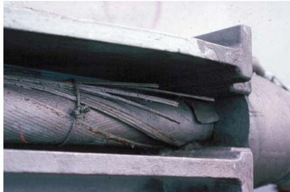
Figure 5: Köhlbrand Bridge at Hamburg: Lower cable anchorage with broken wires
