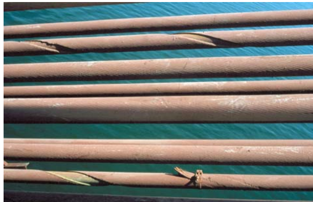
Figure 6: Maracaibo Bridge, Broken Wires
